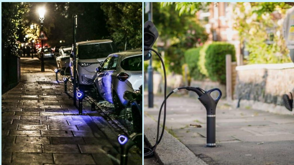
Figure 3.6: Trojan Home chargers
